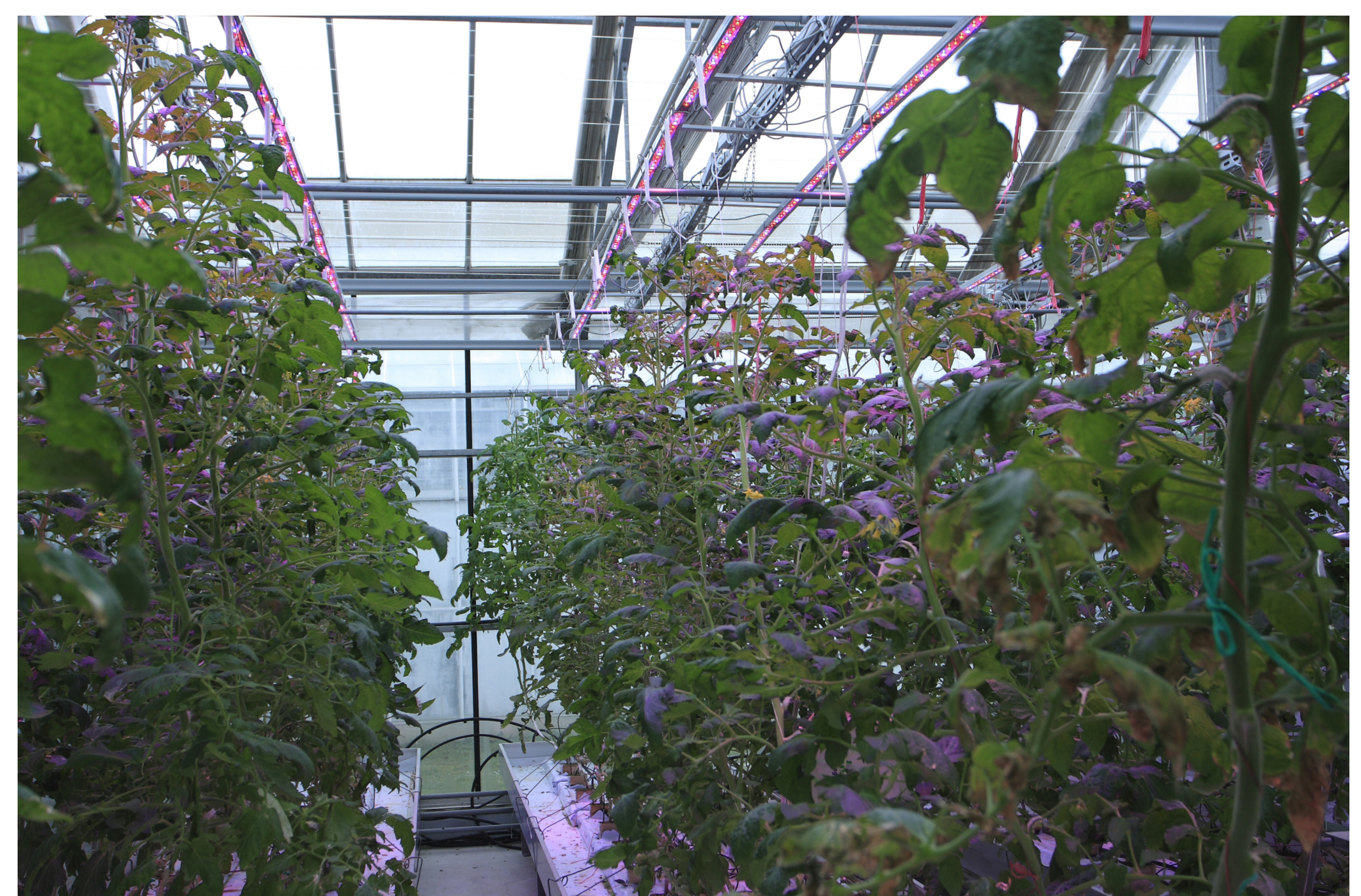
Figure 6. LED lamps in greenhouse
